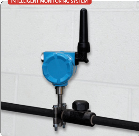
Figure 2. Non-intrusive intelligent monitoring systems can provide immediate notification of faulty steam traps while pinpointing the exact location and nature of the failure.
