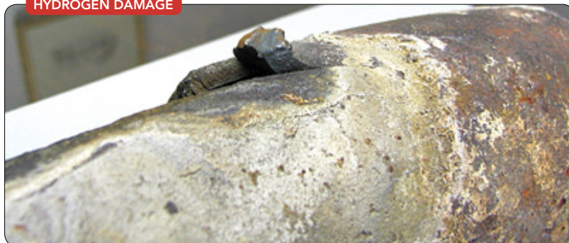
Figure 1. Hydrogen gas molecules penetrate into the metal wall — notice the thick-lipped failure here. Source: ChemTreat.
